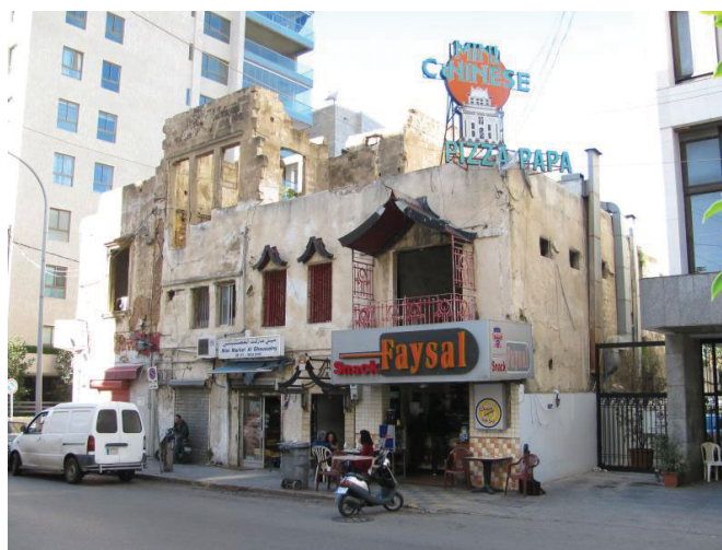
Figure 8.33: Beirut, Lebanon Located in the middle of an upscale neighborhood in Beirut, this food shop is in a building that has not been fully repaired from damage resulting from the 1975 civil war. The restaurant offers diverse foods, including Chinese food and pizza. Steven Damron – mini chinese , pizza papa , faysal – CC BY 2.0.
