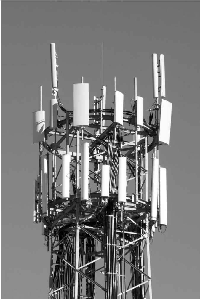
Figure 2.25: The antenna tower of a modern cellular site, supporting several UHF and SHF-band cellular systems.
