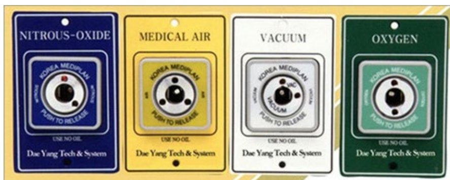
Figure 3.12. Error proofing Medical Gas outlets in hospital incorporating both physical and cognitive constraints.
