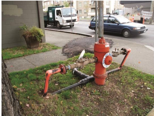
Figure 3-7—Fire hydrant with proper backflow protection
