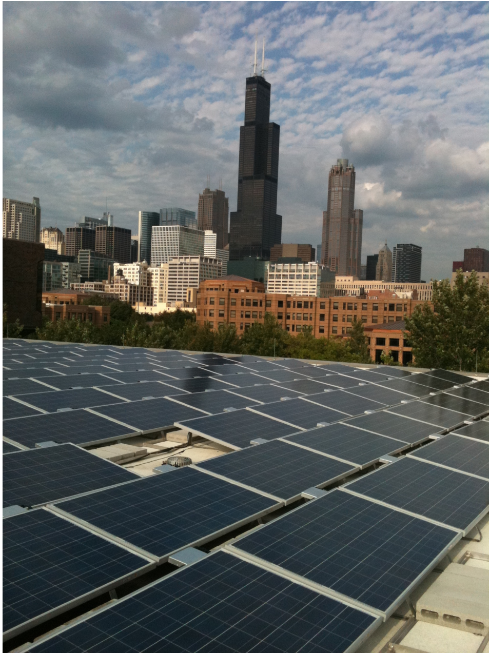
Figure 8.17: Rooftop Solar Installations Rooftop solar installation on Douglas Hall at the University of Illinois at Chicago has no effect on land resources, while producing electricity with zero emissions. Source: Office of Sustainability, UIC 47
