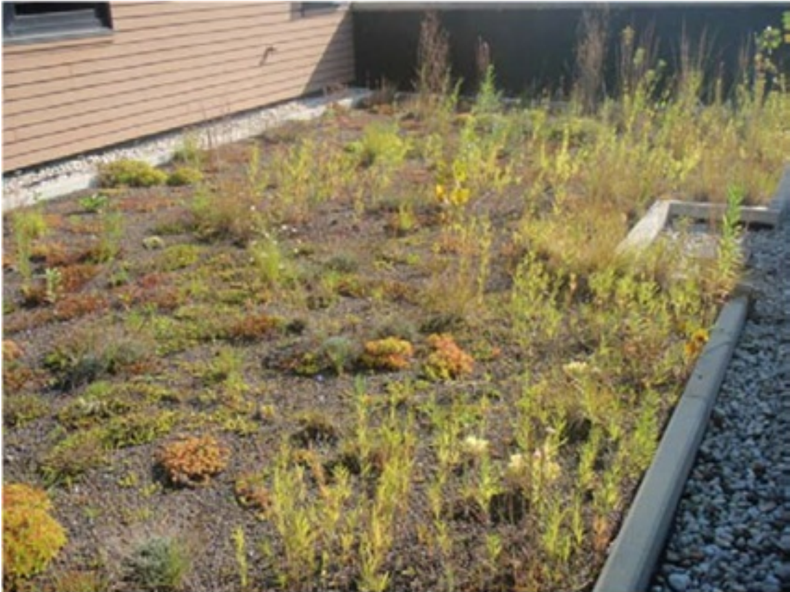
Figure 11.34: A Green Roof The green roof on this police station in Village of Villa Park, Illinois has shallow-rooted plants placed in a thin layer of growing medium installed on top of a waterproof roof membrane. Source: Jaffe, M. et al. (2010) (p. 587), Fig. 13, p. 116.
